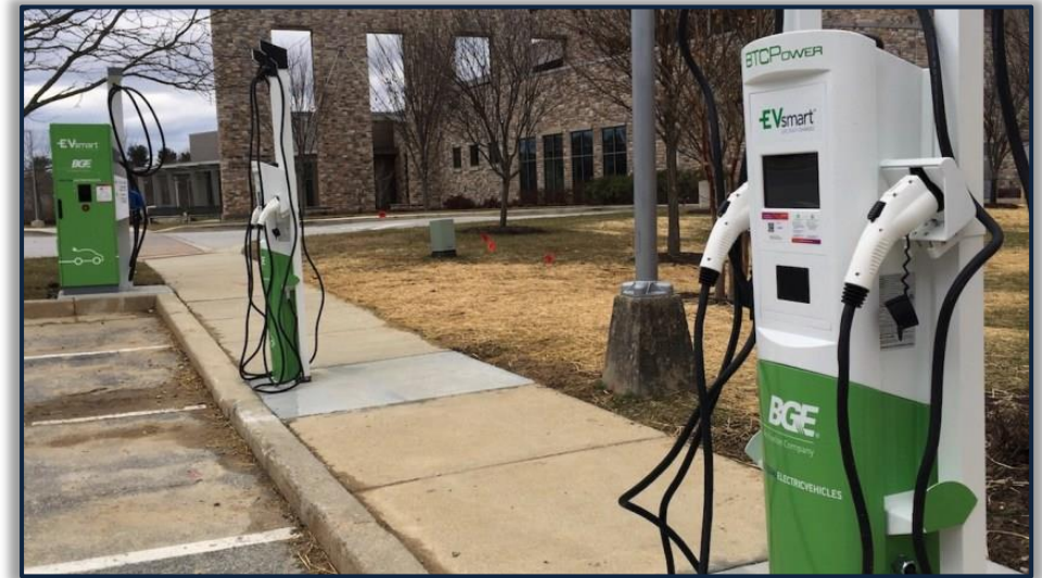
Photo source: https://pluginsites.org/bge-charging-stations-at-library-in-ellcott-city-md/
